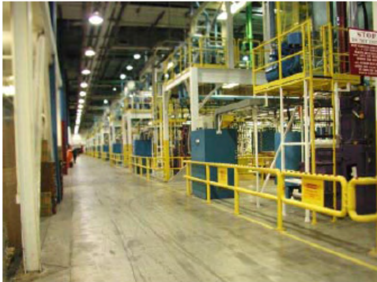
Figure 67. Ten Self-shielded EB Units in One Factory
